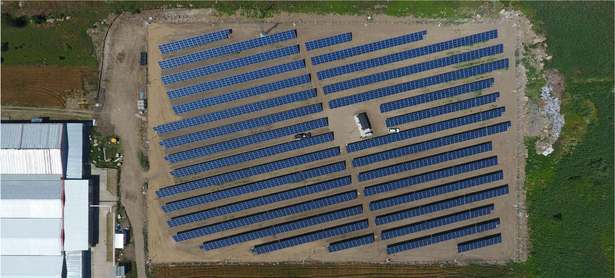
Edirne Giyim Solar Park, 1.16 MWp, Turkey (2018)
